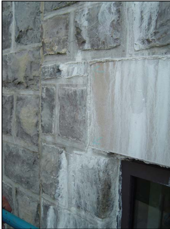
Figure 2. Efflorescence at Masonry Flashing
