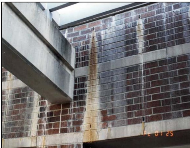
Figure 4. Efflorescence on Brick Masonry Wall from Paver Setting Bed Behind Wall
