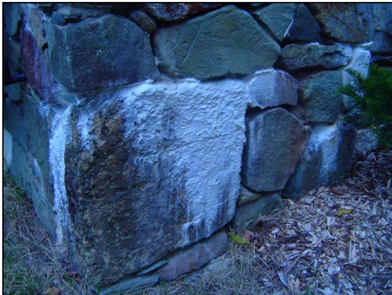
Figure 3. Efflorescence on Stone Masonry Wall
